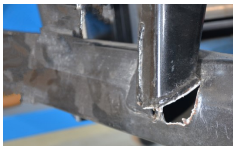
Figure 14. (Scene of local damage)
